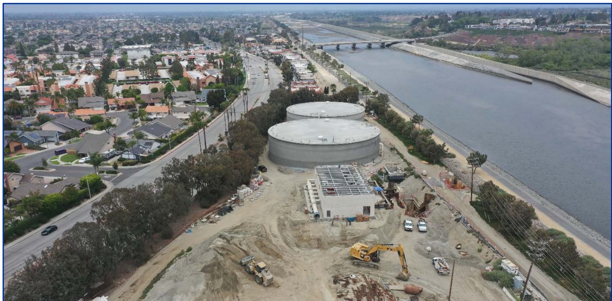
Figure 2-4. OC San Plant 2 Secondary Effluent Flow Equalization (SEFE) Tanks and Pump Station
