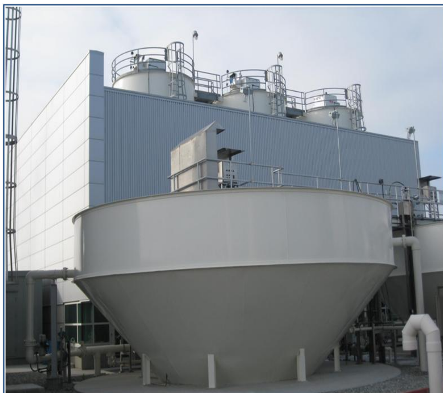
Figure 2-24. Lime Post-Treatment System
