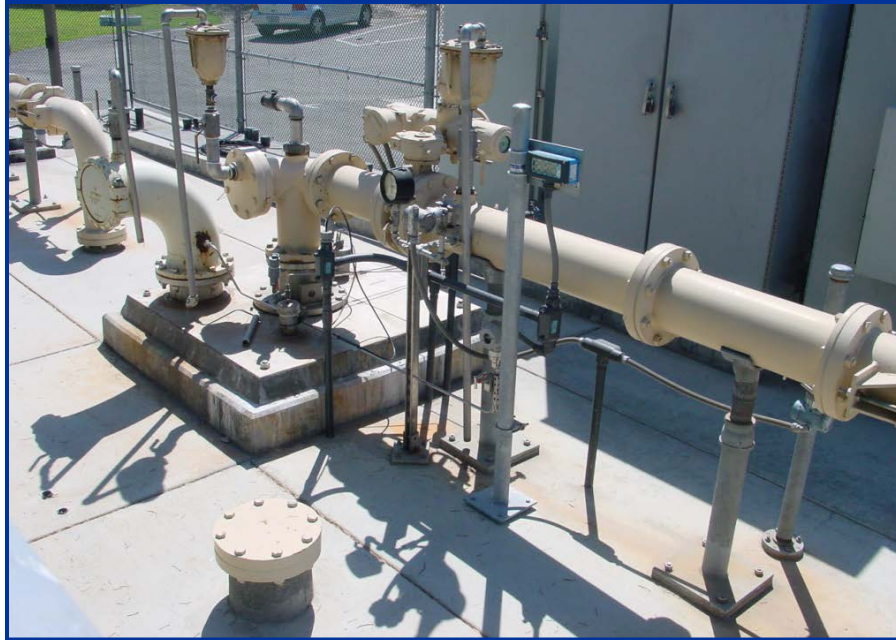
Figure 3-3. Modern Injection Well Site I26
