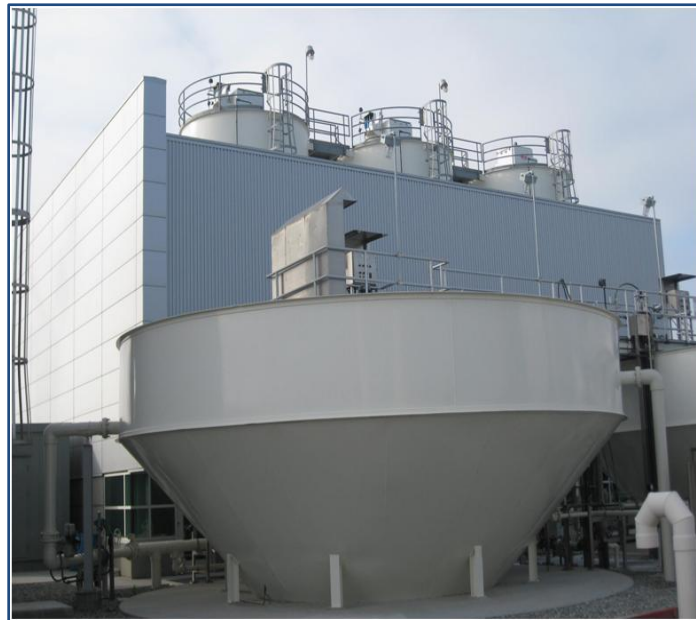
Figure 2-16. Lime Post-Treatment System
