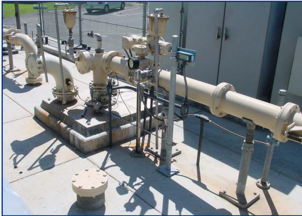
Figure 1-15. Modern Injection Well Site I26
